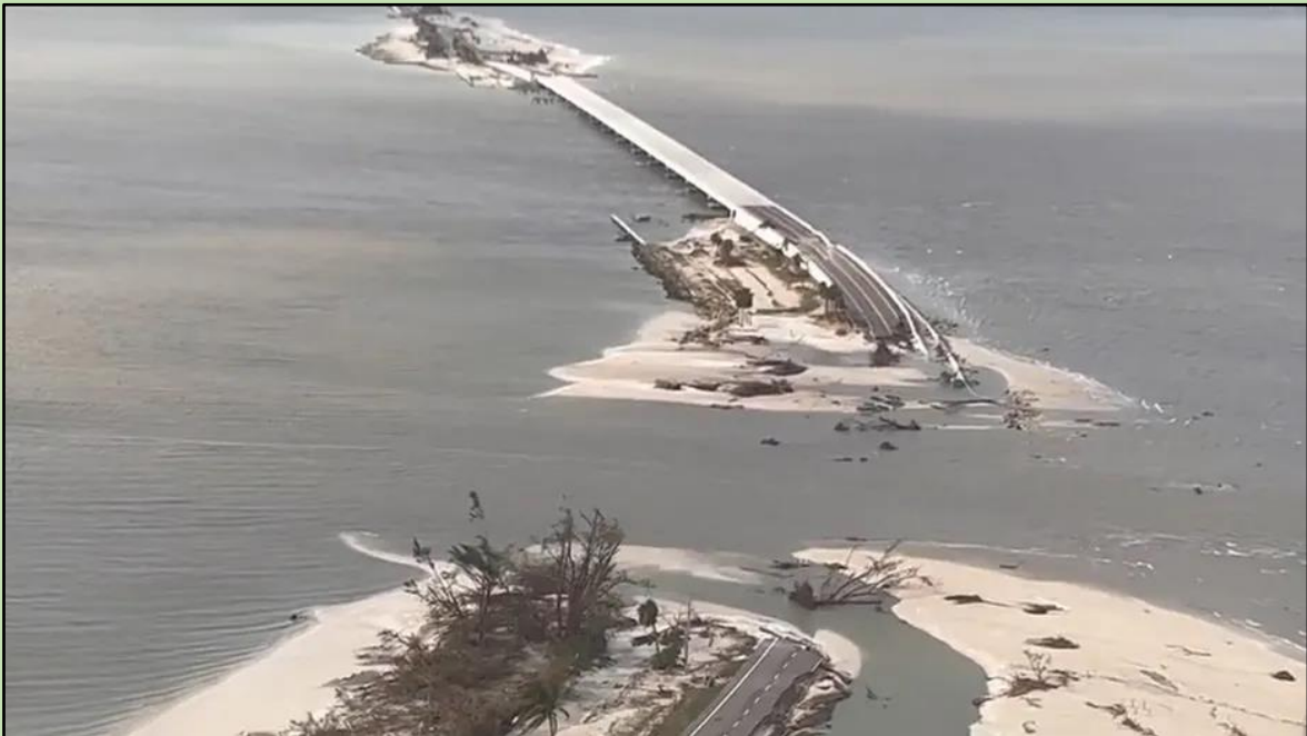
Figure 51. Aerial View of Sanibel Causeway, Destroyed by Ian, Cutting Off Sanibel and Captiva Islands (Reprinted from Fox 13 Tampa Bay; Lee County Sheriff's Office 2022.)
